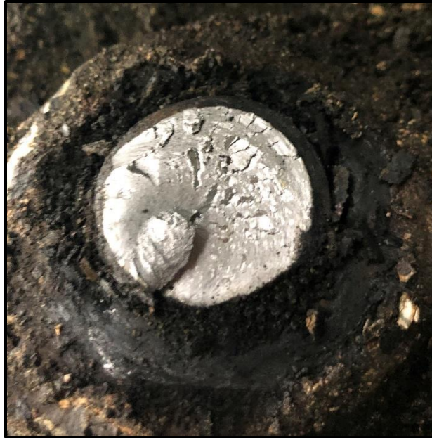
Photo 5: Live Load Shoe Anchor Bolt Sheared
