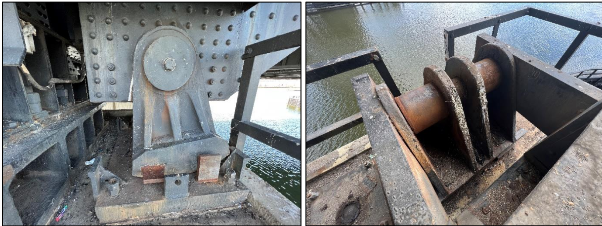
Photo 2: Left - Live Load Shoe; Right - Live Load Shoe Fixed Pin
