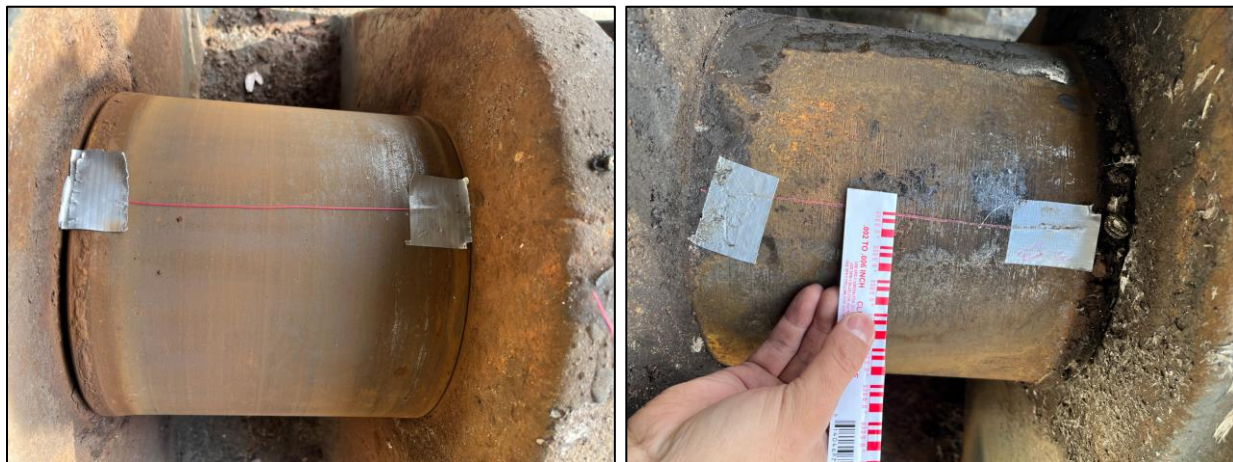
Photo 3: No contact on southwest live load shoe (left) & minor contact on the northwest live load shoe
