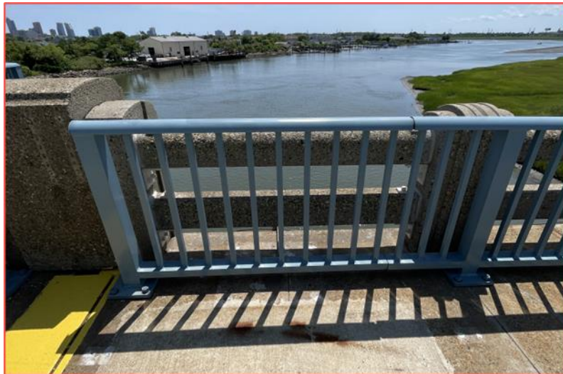
Figure 11: New Aluminum Railing in Front of Existing – Note the original concrete railings are visible
