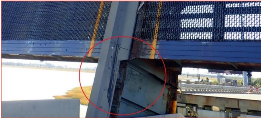
Figure 8: Impacted Aluminum Median Barrier
