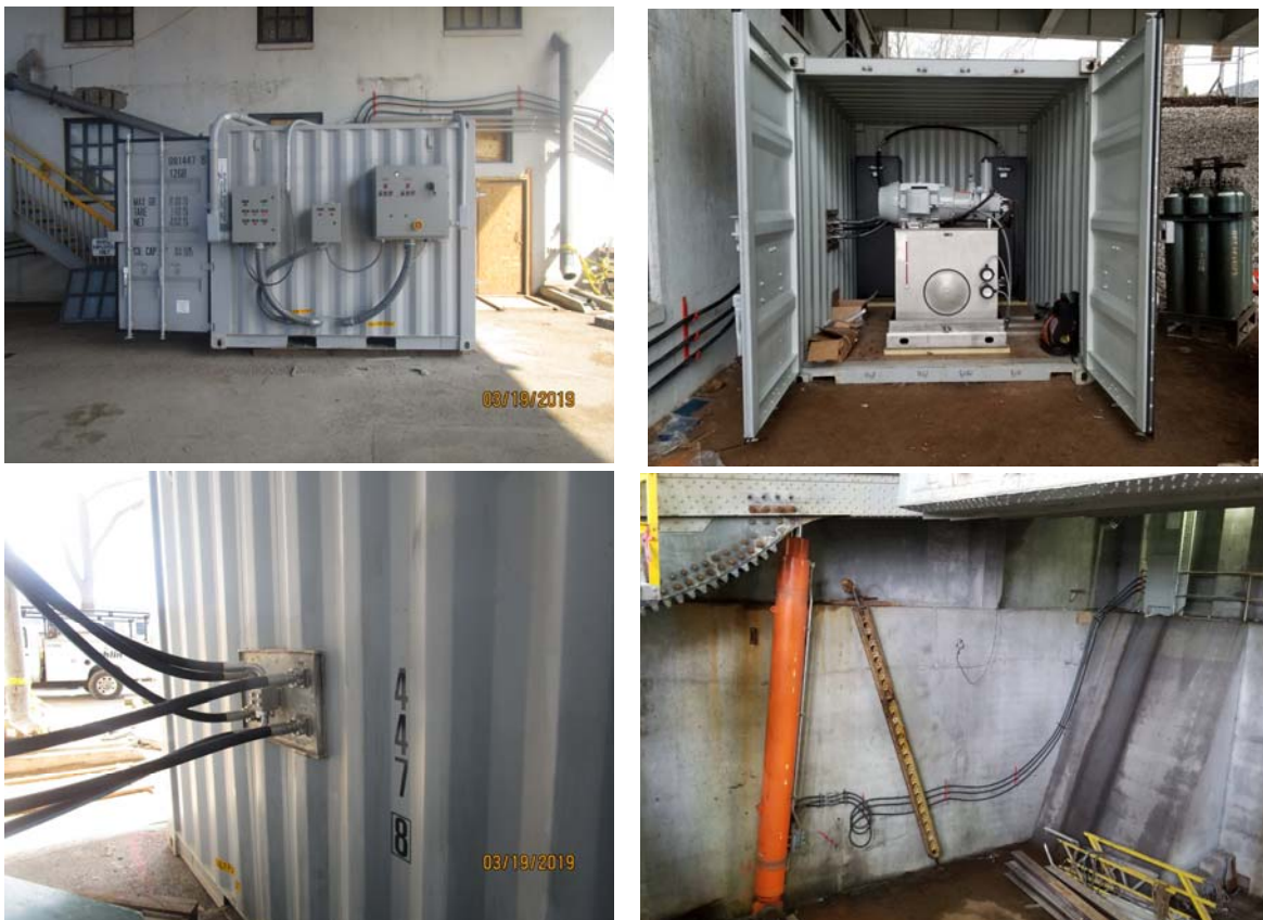
Figure 11 – TOS Hydraulic Power Unit Arrangement and Routing to Cylinders.
