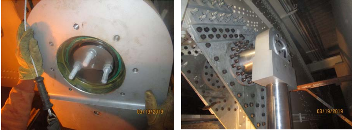
Figure 10 – Fit-up Rod End on TOS Cylinder using Alignment Plug and Final Connection.
