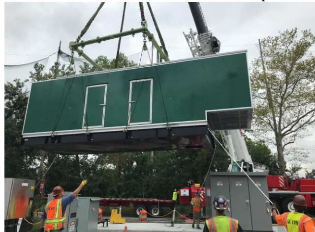
1000 KW generator being installed. Due to size of generator and equipment, the foundation and position were redesigned multiple times during the design phase
