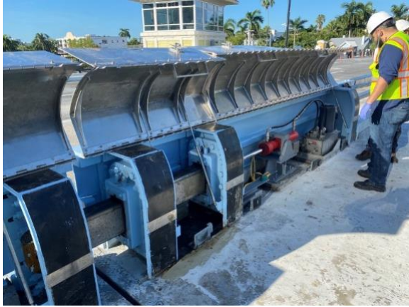
Deck-mounted span lock assembly with hatches open.
