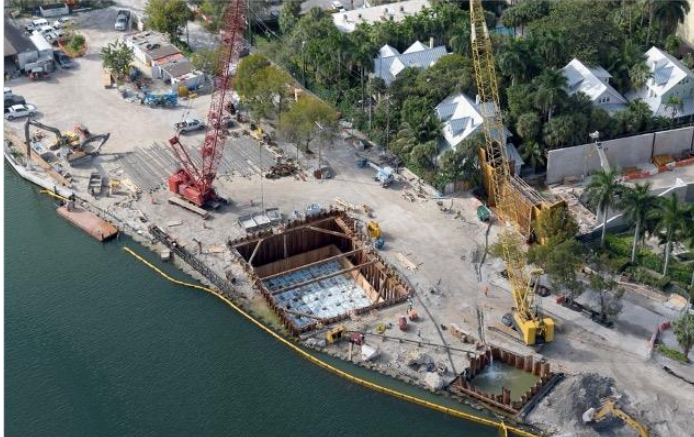
Note the proximity of the adjacent historical structures to the site—especially the abutment and walls.
