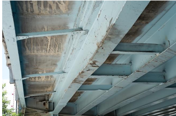
Vehicle impact damage to the 1929 structure approach span girder flanges.
