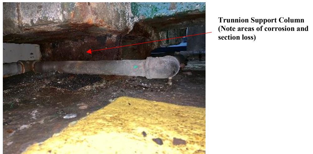
Figure 6 - Trunnion Steel Support Requiring Repair
