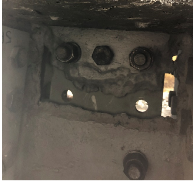
Figure 13 - Northwest Trunnion Support with 100% Section Loss
