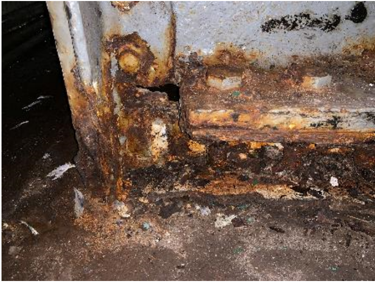
Figure 4 - Pinion Support Area Requiring Repair
