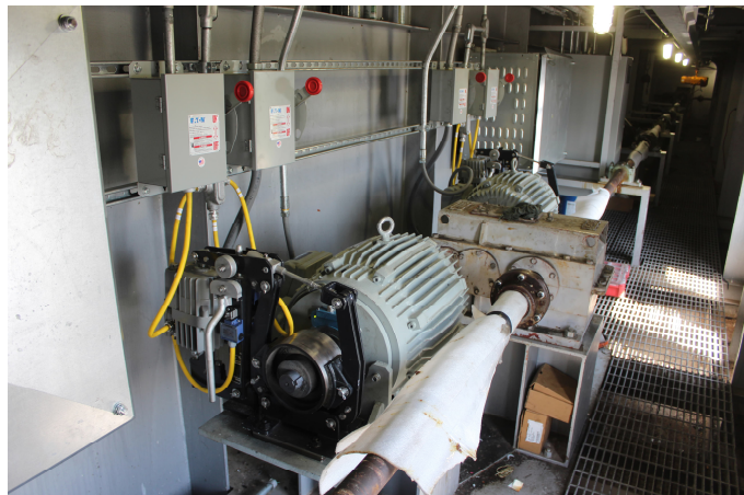
New Span Drive Motors
