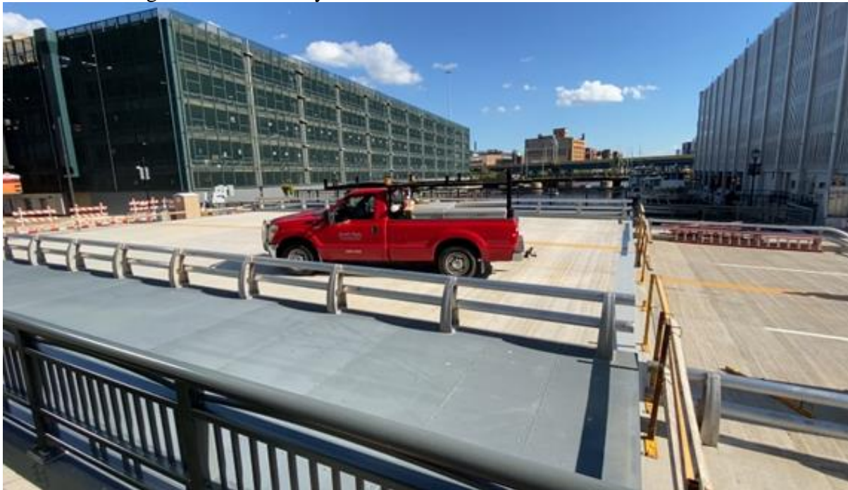
Photo 20: Field Testing Uneven Cylinder Loading with a Truck Parked on the Span
