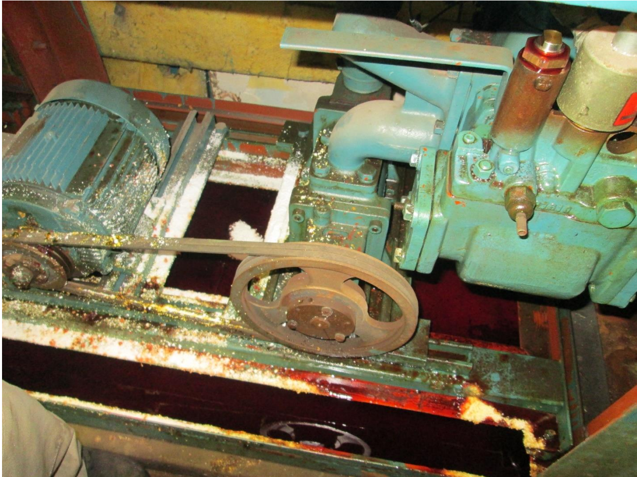
Photo 6: Leaks at the existing Hydraulic Power Unit
