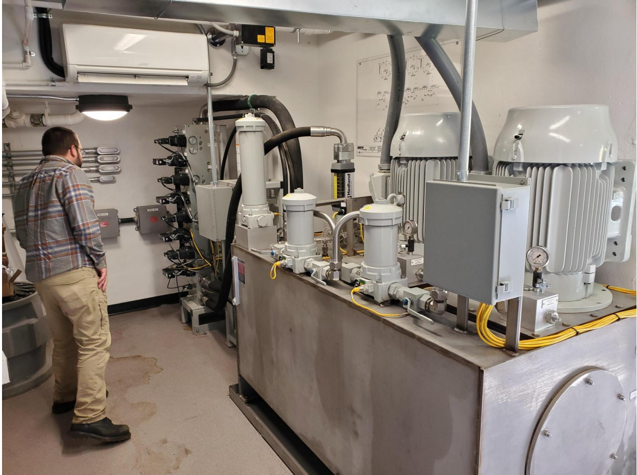
Photo 14: Hydraulic Power Unit
