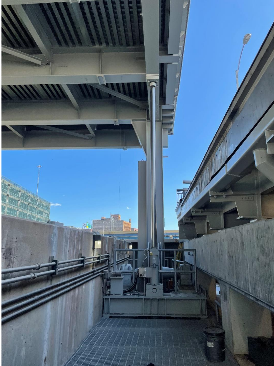
Photo 11: Hydraulic Cylinder with the Span in the Fully Open Position
