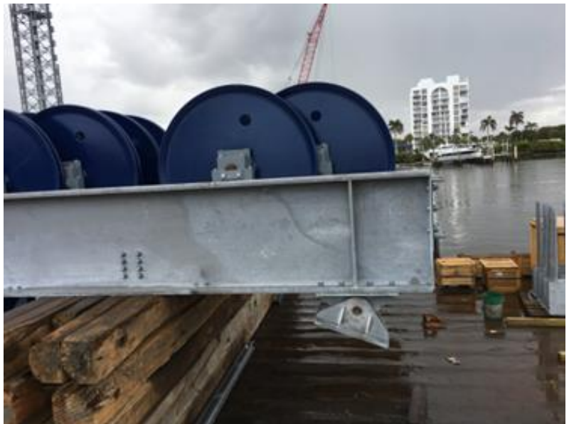
FIGURE 23: Crosshead/sheave pallet and bearing
