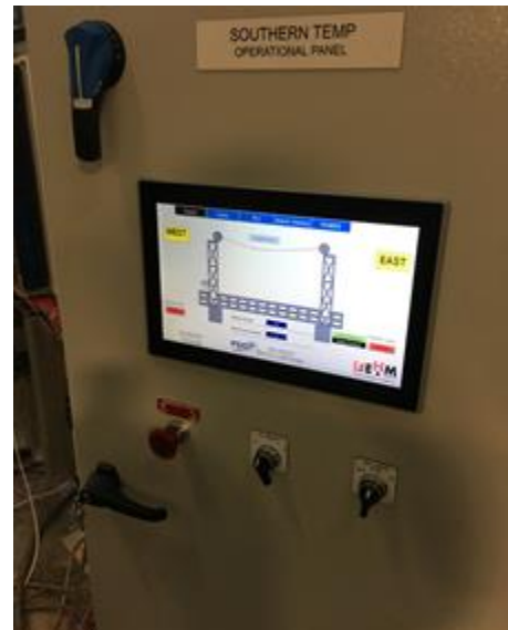
FIGURE 37: Typical HMI panel
