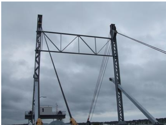
FIGURE 52: Masts and frame
