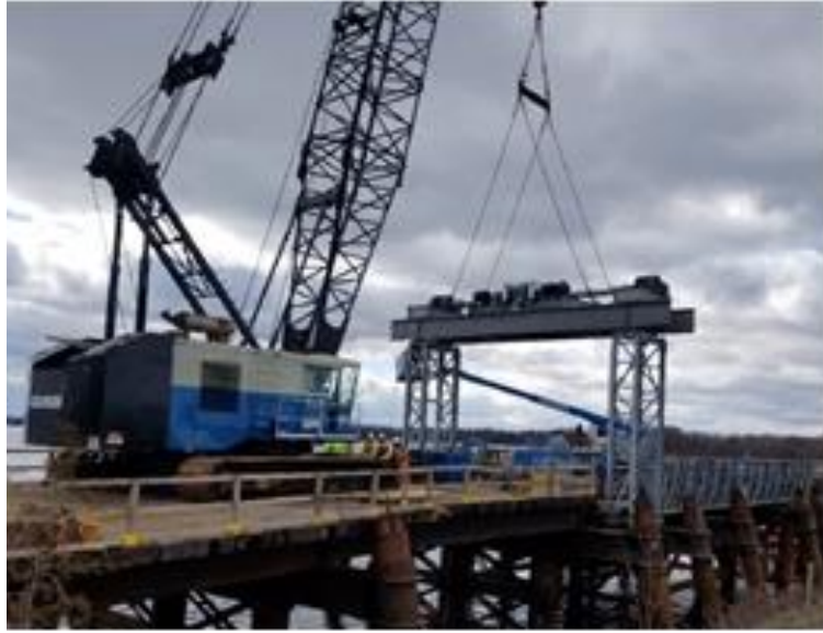
FIGURE 56: Pre-assembled gantry/machinery pallet
