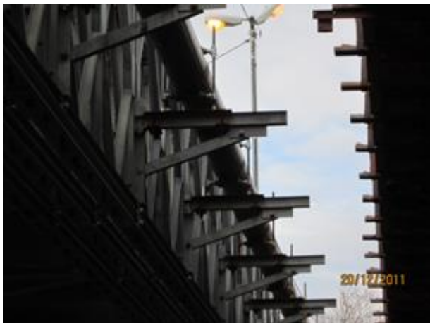
FIGURE 14: Footwalk Bracket Supports
