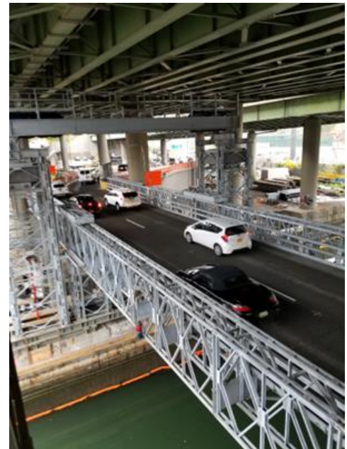
FIGURE 35: Unionport, NY Site conditions
