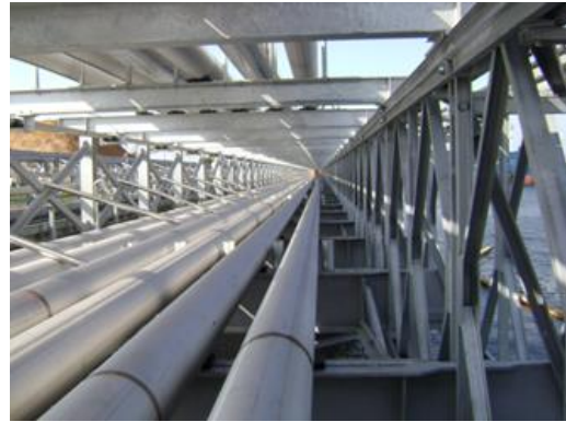
FIGURE 17: Custom Pipe Trestle
