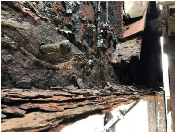
Figure 1: Deteriorated Bottom Flange
