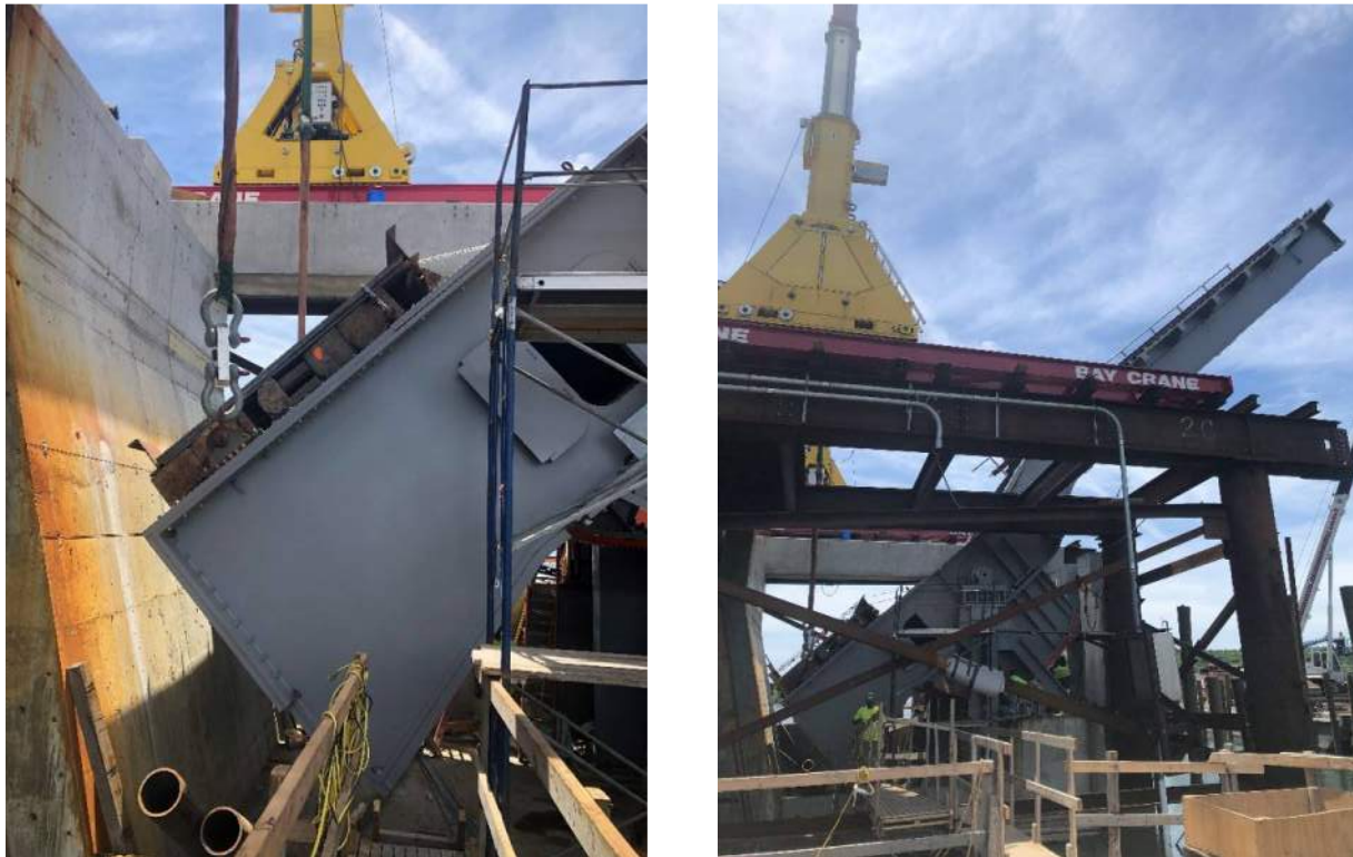
Figure 18: Two views of the leaf being raised via the gantry. The view on the left shows the temporary ballast for stage 2 balance.
