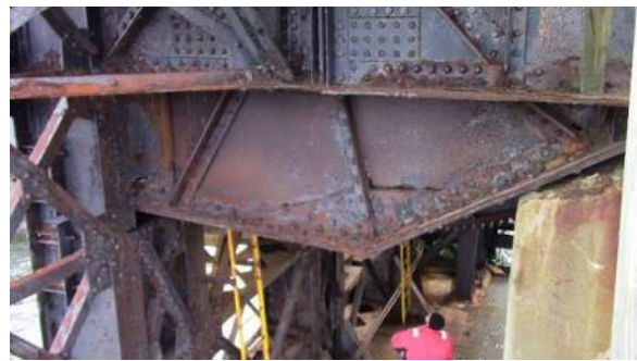
Figure 2: Bascule Girder Web Deterioration
