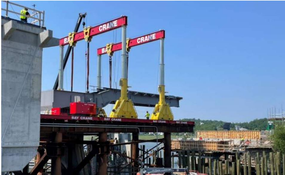
Figure 16: The leaf being moved over the pier via the hydraulic lifting gantries.
