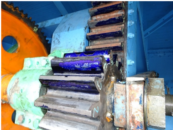
Figure 6: Far opposite rack and pinion contact on the opening face. Machinery secured with temporary bolts.
