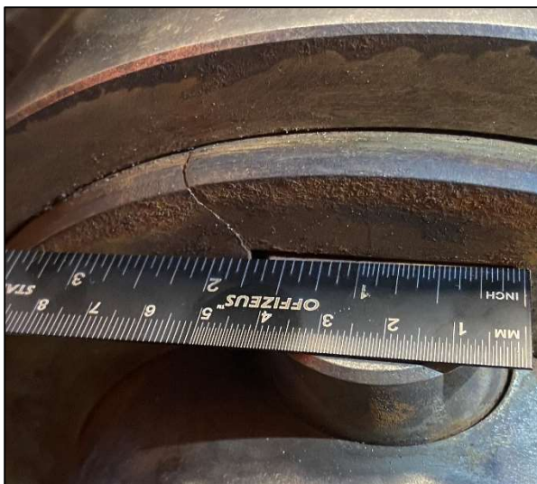
Photo 3: Crack in Coupling Hub
