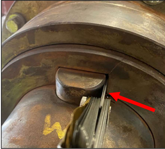
Photo 7: Clearance between west pinion hub key and keyway. Note crack at SW corner
