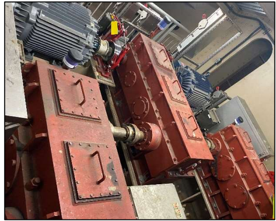
Photo 2: Span Drive Machinery
