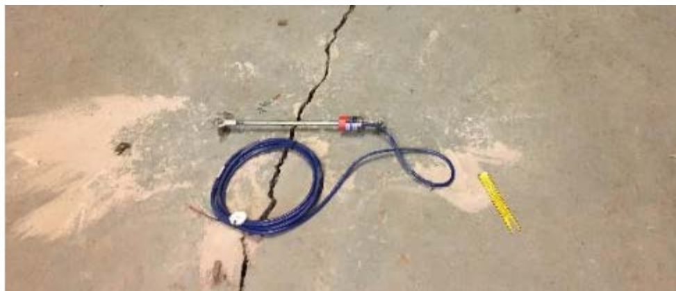
Crack Meter installation inside the SLSMC Electrical Room (total of 8 crack meters installed at various crack locations)
