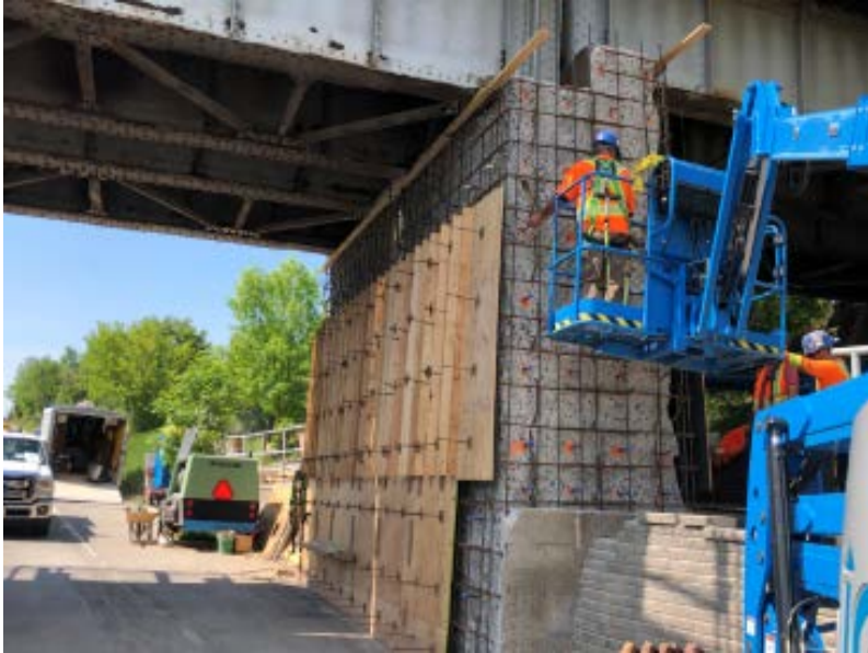
Fixed Approach Spans Center Pier Rehabilitation – southbound lane and trail closed Reinforcing steel and anchors installed, formwork in progress
