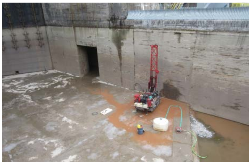
Borehole drilling at floor of Lock 4 East adjacent to Center Monolith (West similar on opposite side)
