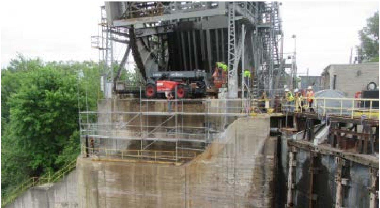
Preparations for the concrete repairs of the East Monolith Bridge 6 East raised, existing front tread and track plate segment removal in progress
