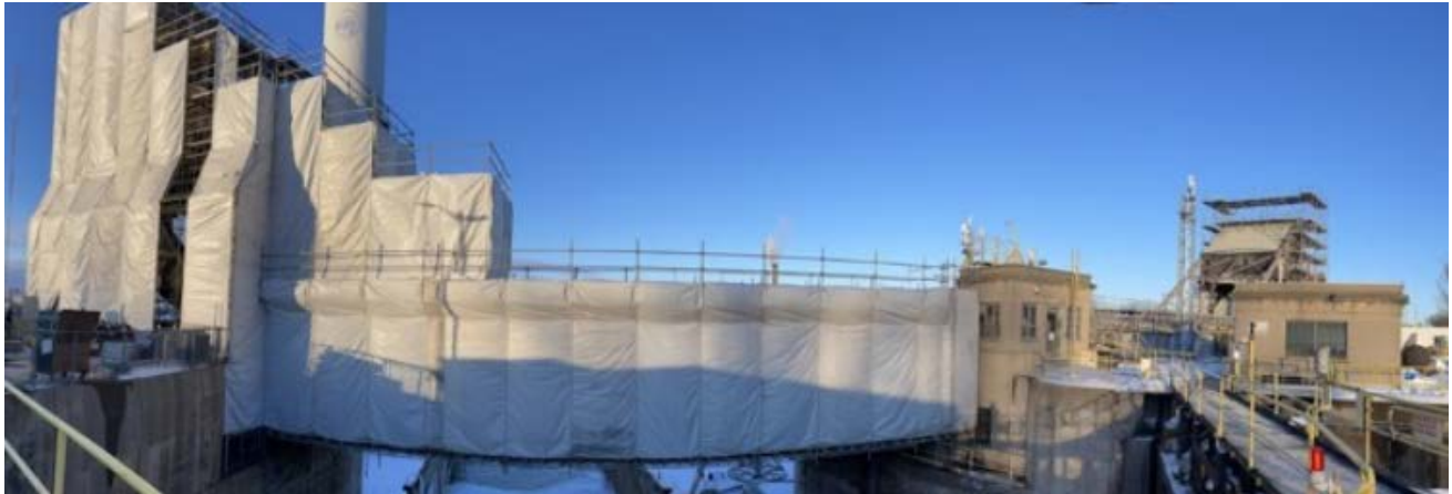
Bridge 6 West – Scaffolding and Enclosure installed for painting and counterweight re-facing Bridge 6 East – Scaffolding installation in progress - (looking North)
