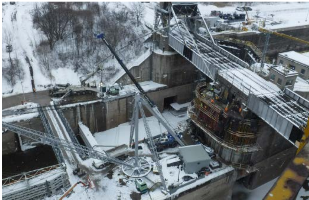
Bailey bridge connecting Lower Lock 4 East with the center wall bullnose Concrete pour at the center monolith wall
