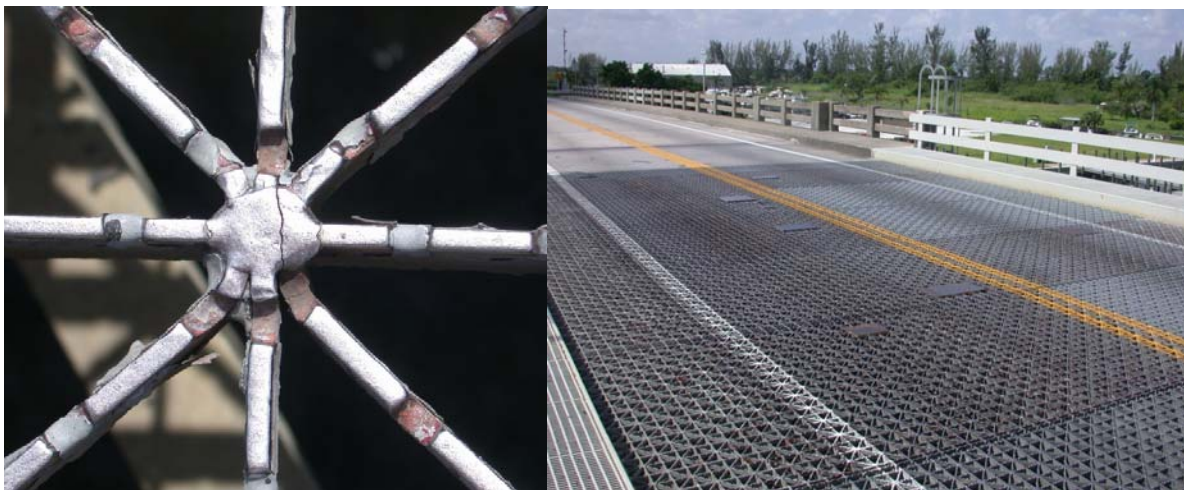
Figure 3. Typical Steel Open Grid Deck Fatigue Crack and Welded Repairs
