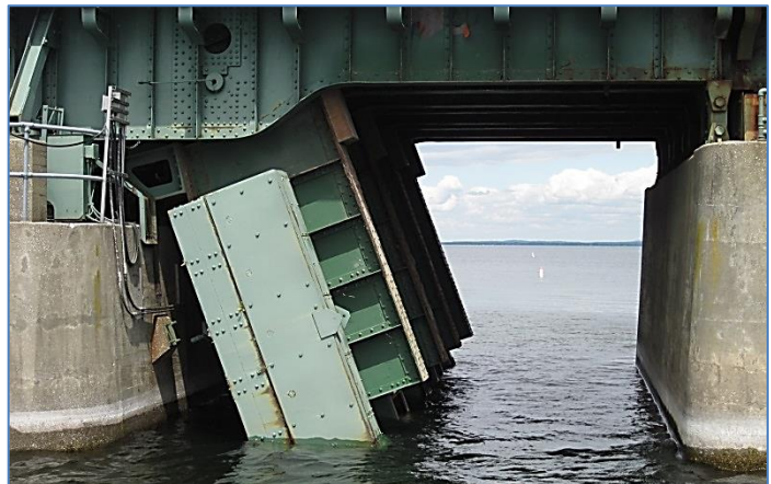
View of the existing span in the open position. Note counterweight partially submerged in the water.
