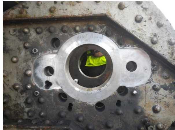
Photograph 9 - 2 nd Link truss gusset plates after initial machining. Note the original keyway removed from the bores and facing in the area of the new gusset sleeve flanges
