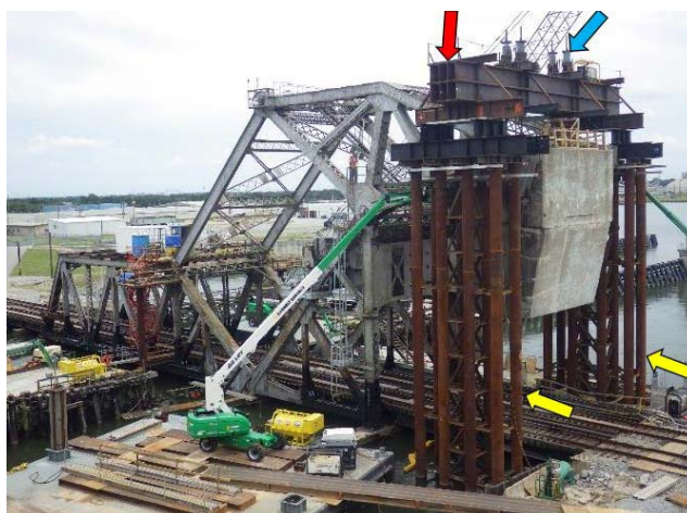
Photograph 4 - Temporary counterweight support structure. Note the pile structure on each side of the counterweight (yellow arrows), the four main double stacked W36x395 beams (red arrow), and the hydraulic jacks and Williams Rods (blue arrow)
