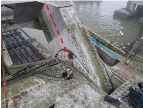
Photograph 1 - General view of the lakeside 2 nd Link Joint. Note the counterweight link centerline (red dashed line) and operating strut centerline (blue dashed line).
