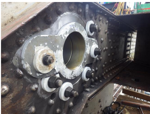
Photograph 10 - New gusset sleeves, shear insert plugs and thru bolts installed at the 2 nd Link joint in preparation for installing the main pin.
