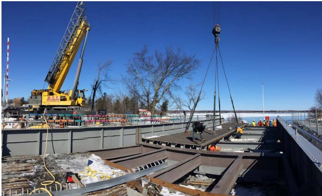
Figure 4: Installation of OSD panels to the existing twin girders during winter – Kingston
