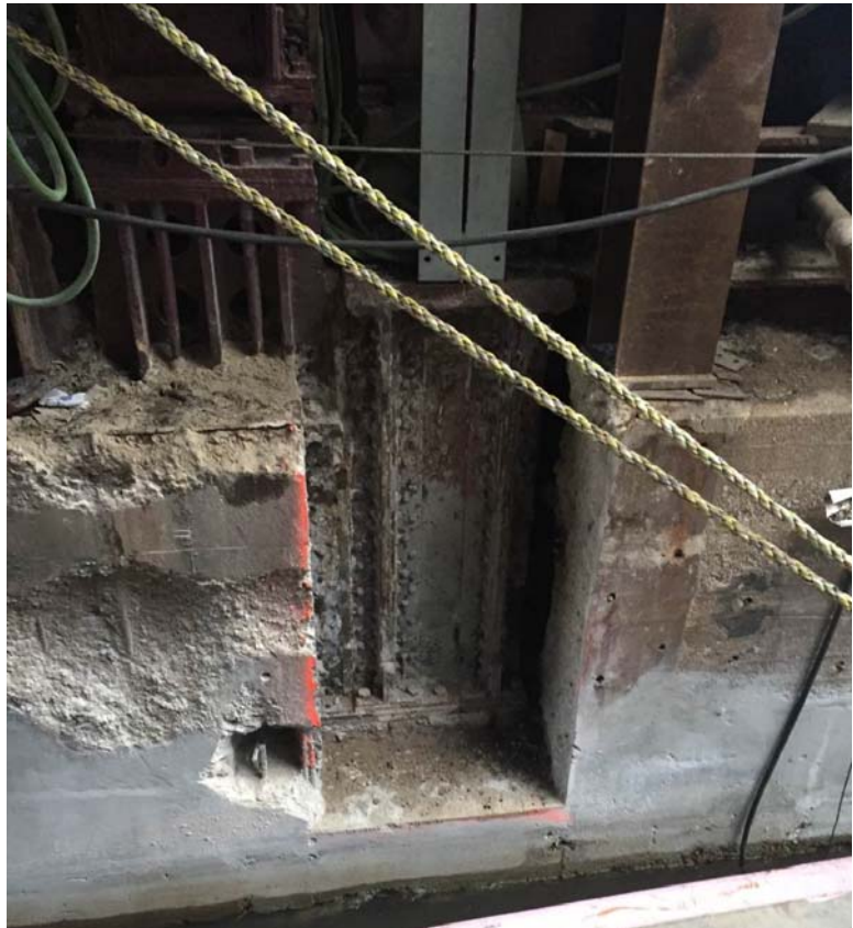
Figure 6: Mined out River Wall with Longitudinal Girder, Live Load Bearing and Bridge House Column
