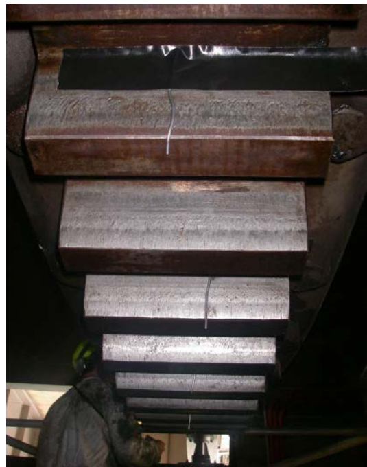
Photograph 6 – Lead solder used to determine backlash during operation
