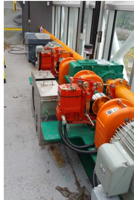
Figure 5: Span drive machinery (primary reducer in center of photo)
