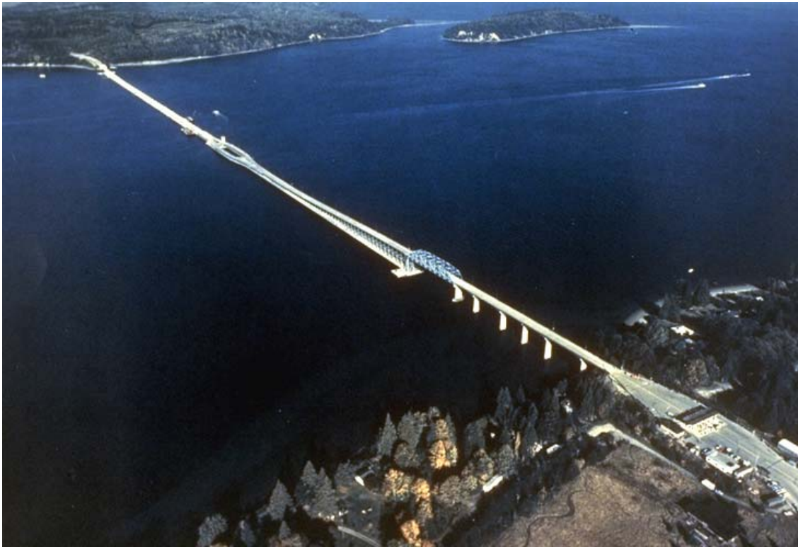
Figure 3 – Aerial Photo Showing Existing East Half (Near) and New West Half During Stage 1
