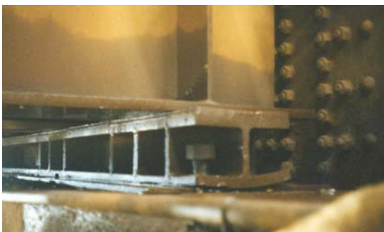
Photograph 2: Existing approach span bolster beam. Note the deformation in the bottom flange.
