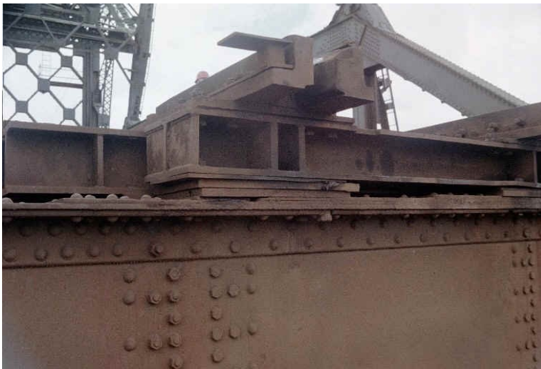
Photograph 3: The old rail joints sat atop a steel tie that was supported by several shims of various sizes and thicknesses.
