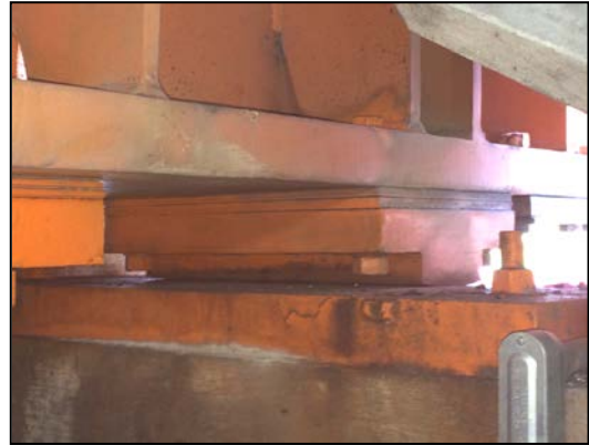
Photograph of a Typical Forward Live Load Bearing of a Double-Leaf Trunnion Bascule
