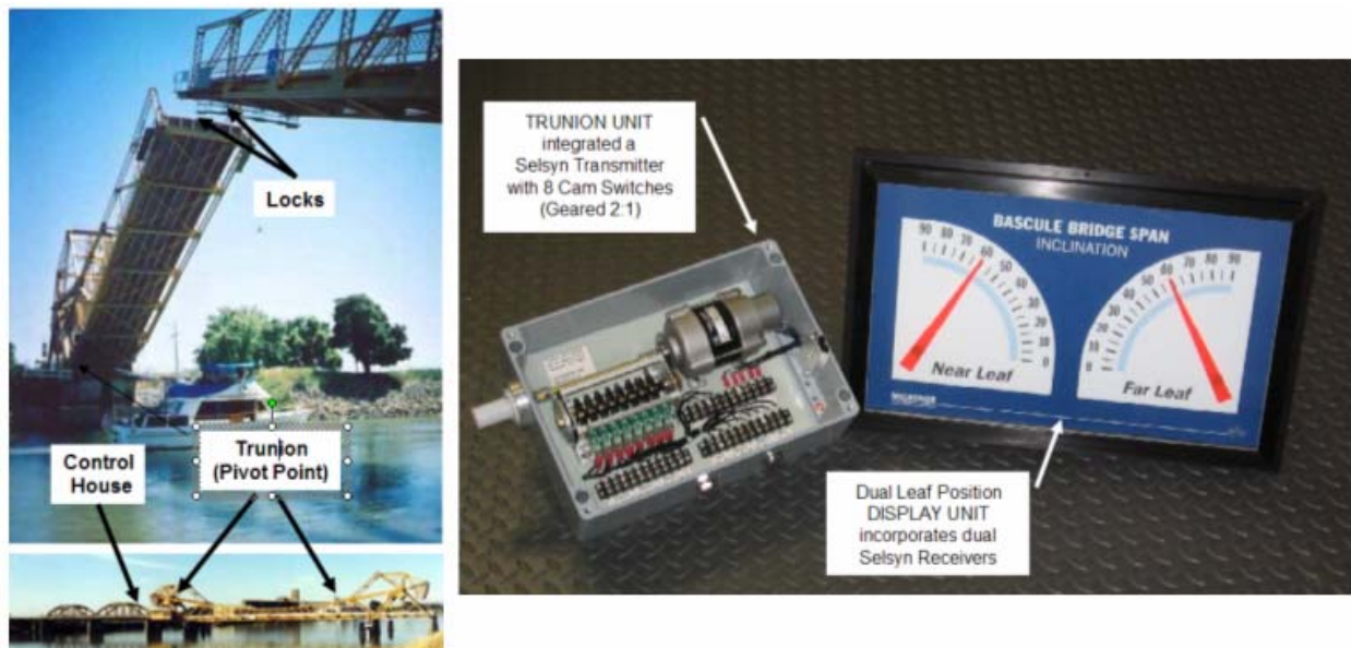
Figure 7. Sacramento area bascule bridges were upgraded with new selsyn-based position display system (with LED backlight) and new rotary limit switch controls.
