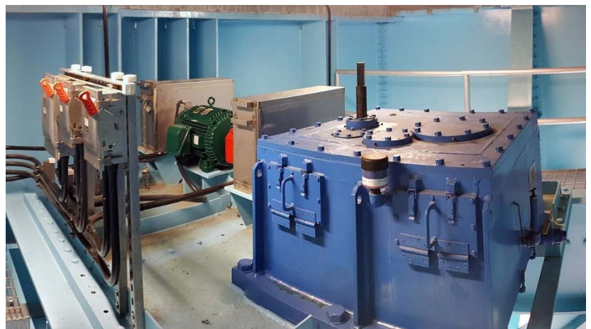
Span Operating Motor, Brakes and Reducer on Machinery Platform
