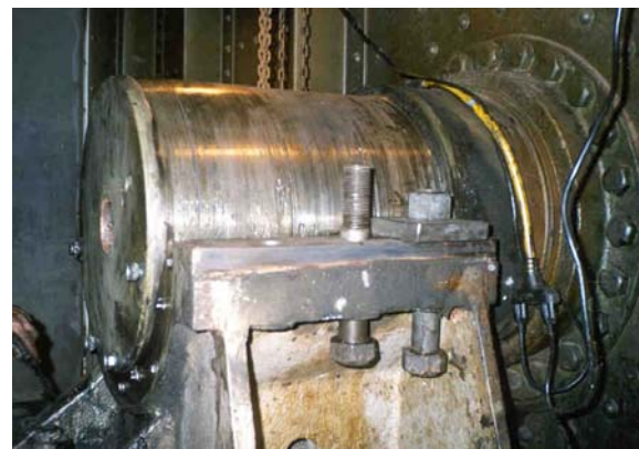
PHOTO 2: Condition of South Trunnion at Wappoo Creek Bridge prior to machining.
