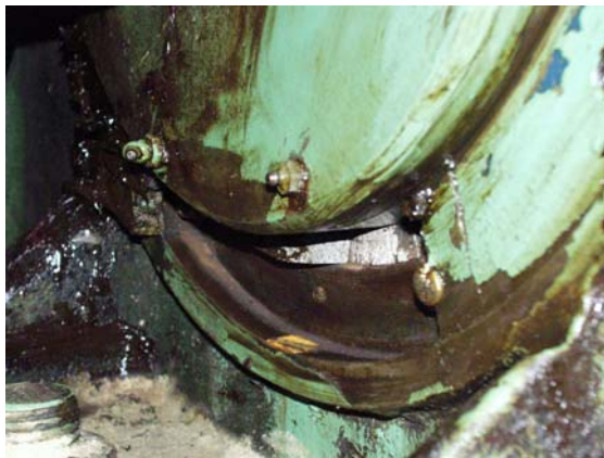
PHOTO 6: West Trunnion of Wrightsville Beach Bridge showing cracked bushing and section of flange missing.
