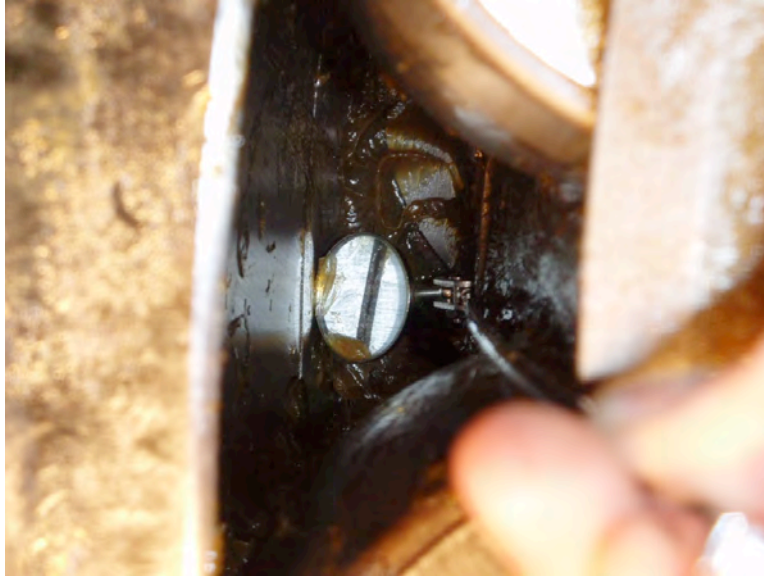
Photo 3: SW Outboard Location, Outer Ring, Crack Location
