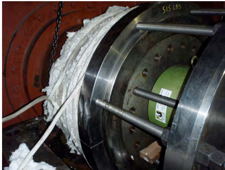
Photo 4: SW Outbound Bearing, Heating Coils and Puller Device
