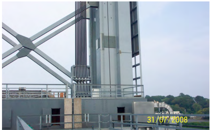
One of the two cable chases on the lift towers
