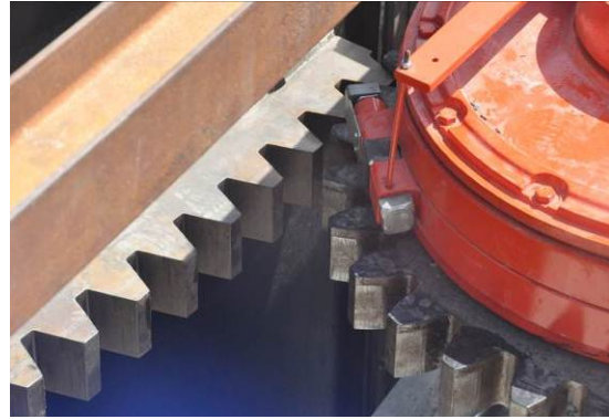
Drive Gear and Rack Gear on Sector Gate
