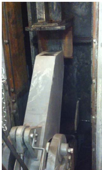
Dogging arm with actuating cylinders as gate is about to come to rest
