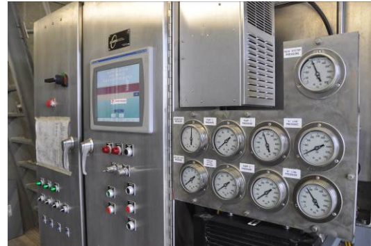
Vertical Lift Gate Hydraulic Power Unit with Control Panel
