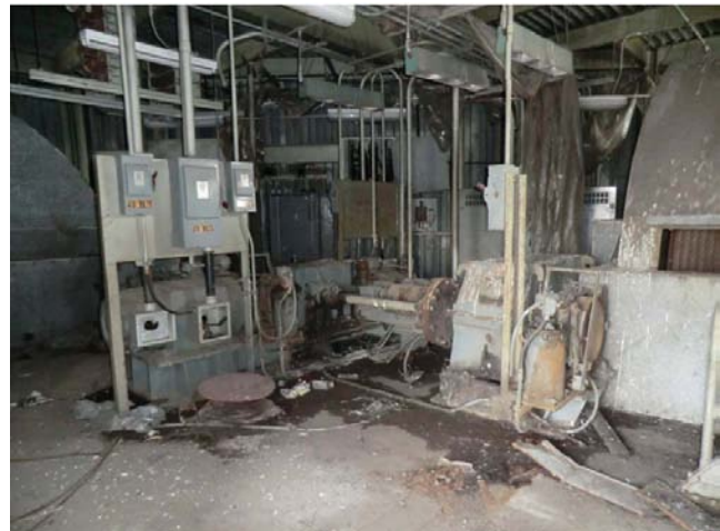
Tower Control Room showing main motor, reducer and main sheave
