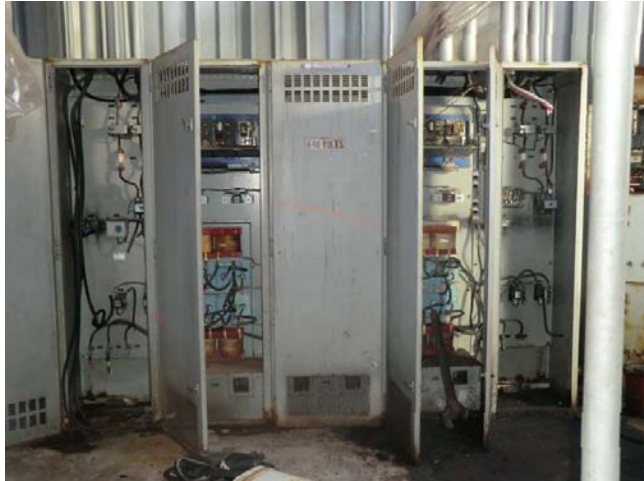
Condition of Motor Generator Set in Bridge Tower
