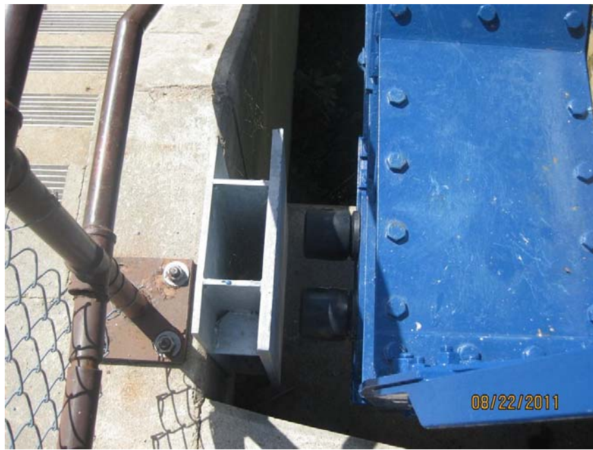
Photo 5: Energy Absorbing Bumpers at the Channel Open Position
