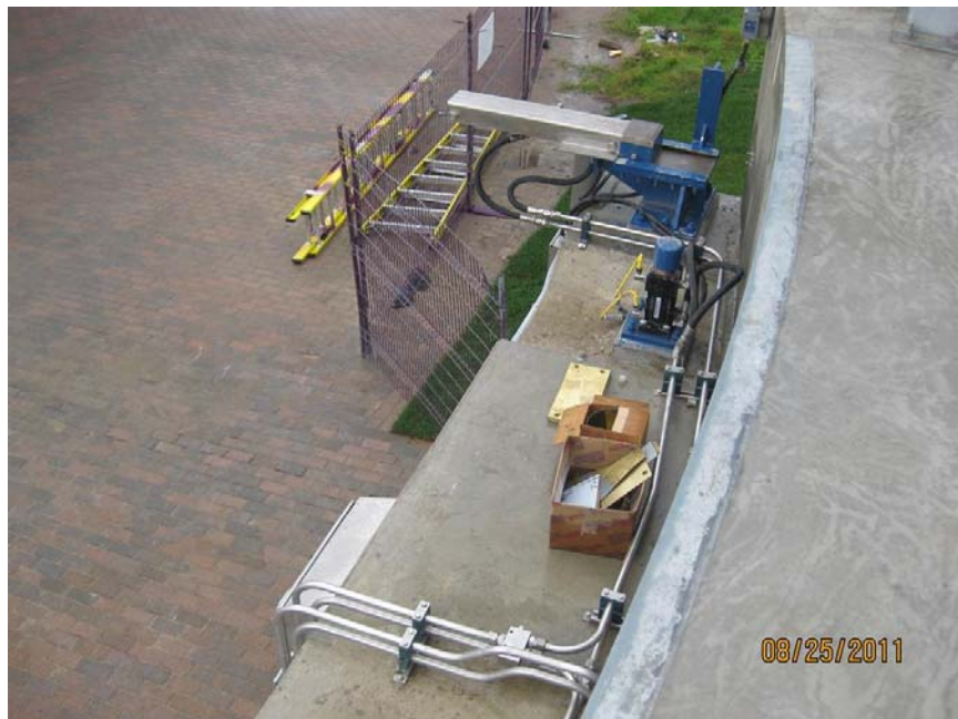
Photo 4: New Installation for the End Jack and End Wedge including the Hydraulic Piping
