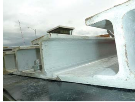
CAPTION: Cracked FRP Panels
