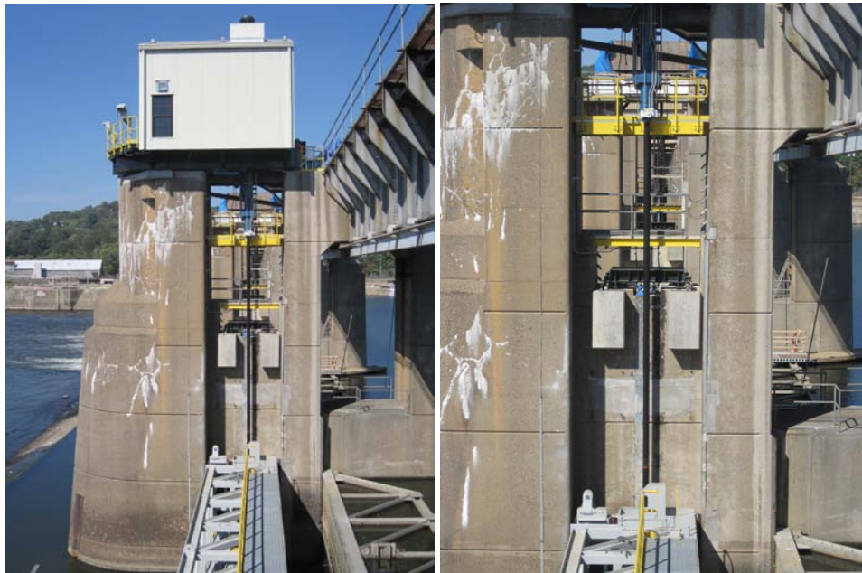
Figure 5. Gate lift hydraulic cylinder
