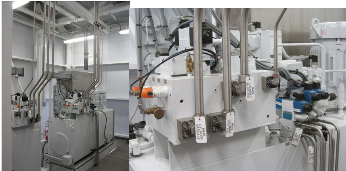
Figure 9. Hydraulic power units
