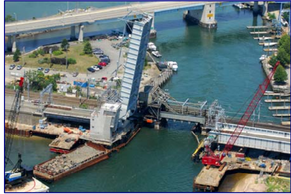
Figure 1. The New Niantic River Bridge and the Old Bridge, Approximately One Month before Opening for Service
