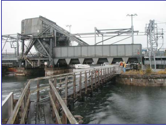
Figure 2: The Old Niantic Bridge in 2004. Note the Large Segmental Girder on which the Bridge Rolls Back During Opening. Note the Movable Catenary Unit (MCU) of the Rail Electrification at the Left.
