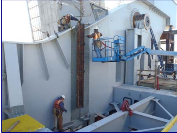
Figure 6: Bolting the Splice between the Bascule Span Rear Portion and Forward Leaf during Float-In
